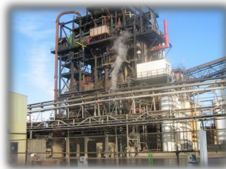
Chemical waste gasification plant (ATM-NL 1998-2013)
