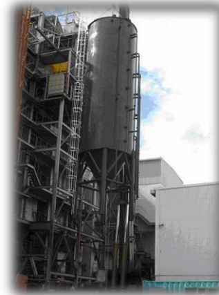
Liquid waste storage tanks (Thailand)
